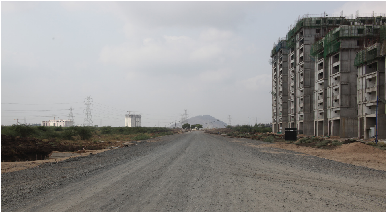
Figure 2. Unfinished infrastructure and housing in Amaravati. May 2019. Photo by Author.
